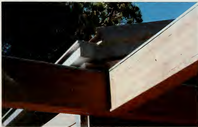
Detail of Microlam beams meeting extraordinary roofing and sheetmetal work. Photograph: Frank Folsom Smith
